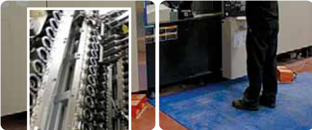
Two NINE Axis Machines installed and running at Mill Close, with 300 tool stations per machine
